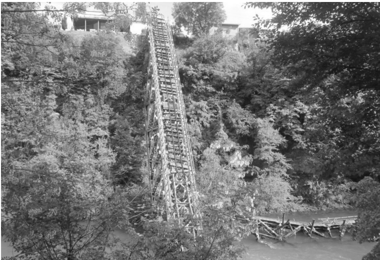
Destroyed Neretva Bridge, Jablanica
